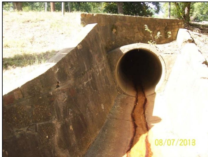
Photo 3 – South System 48" RCP outfall to concrete lined channel north of E. Kay Street
